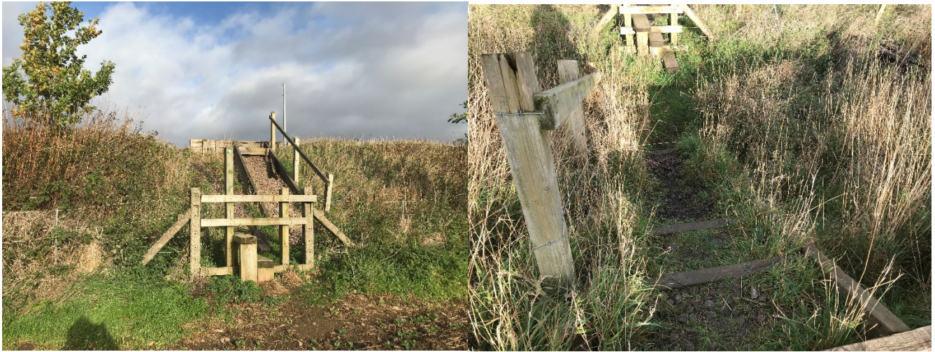
Routes onto the Oxcroft Branch Line where the steps have disintegrated, and a steep stoned embankment is difficult to access.
